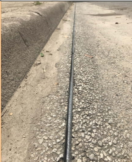
Fiber w/ insulation on top
