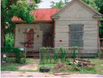
The need for effective enforcement of demolition by neglect and other city code provisions is a significant concern among several stakeholder groups.
