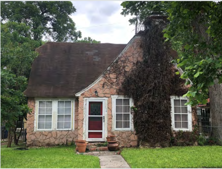
Figure 4.3.2. Example of a door that has been previously replaced with an inappropriate non-historic door that does not fit the style and period of the house. Replacement of this door with a more period-appropriate door is recommended. Source: Photo by HHM, 2021.
