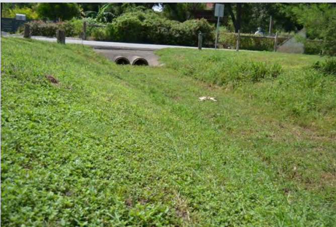
Figure 2.2.5. Example of an earthen swale leading to a concrete culvert that allows two desagues (drainpipes) to allow water to flow beneath the roadway. Source: Photo by HHM, 2021.
