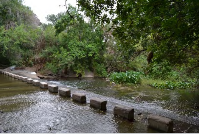
Figure 2.2.4. Example of a low-water crossing in the River Road Historic District. Source: Photo by HHM, 2021.
